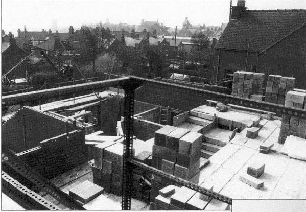
Family First building eight flats for elderly people in Mapperley after demolishing a worn-out house in 1974
